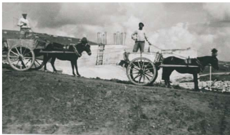
Fig. 120. A transportation vehicle at the time of the construction of the TRINITA' embankment dam (1956)
