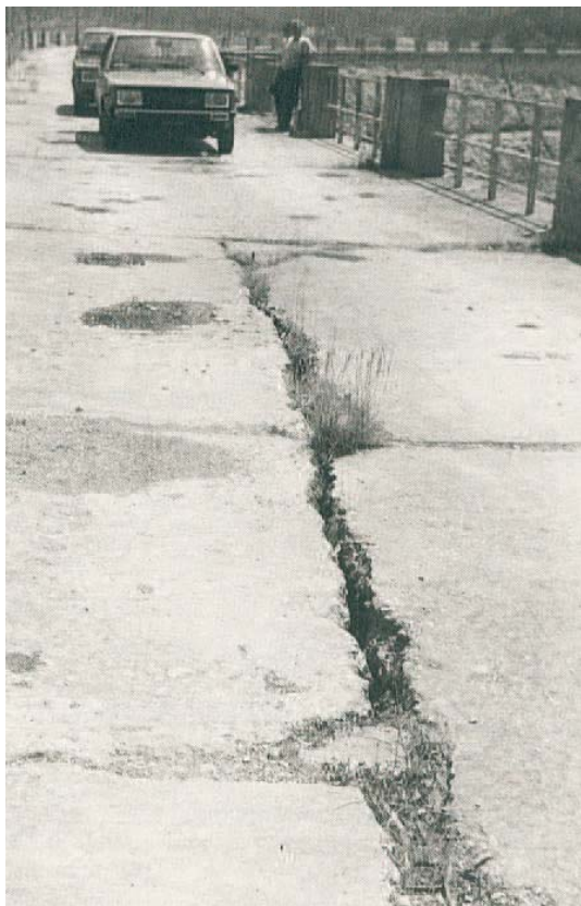
Fig. 110. Longitudinal cracks at the crest of the old DISUERI dry masonry dam after 50 years of service [35]
