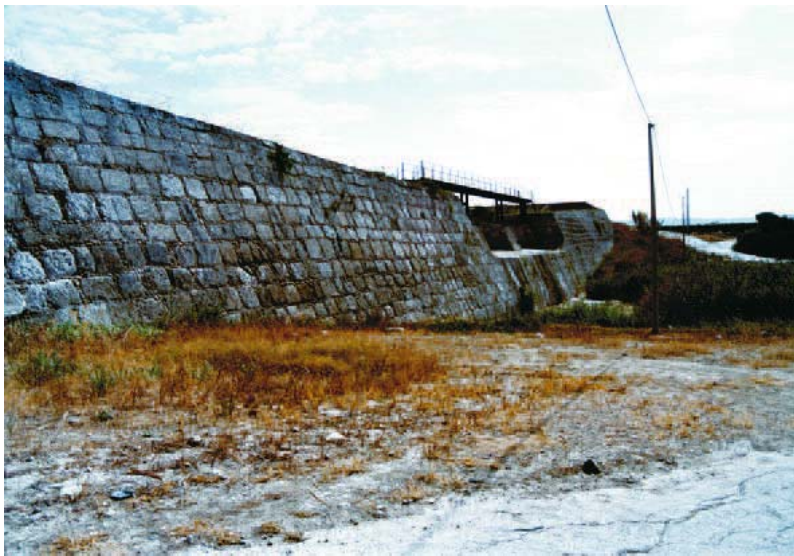
Fig. 29. The GROTTICELLI masonry weir on the Gela River in Sicily, built in 1563 and designed by Architect Carlo Cadorna (photo by C. Gambino)
