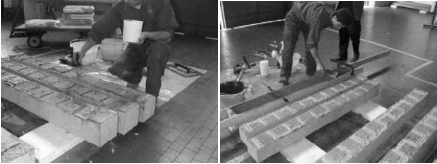
Fig. 1. Restoration phase, anti-corrosion treatment of the irons (a) and volume reconstruction (b)
