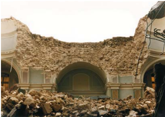
Fig. 42. The soft calcarenite placed in a random fashion in the masonry of the San Corrado church at Noto which failed without premonitory evidence in March of 1996 (photo by V. Jappelli, 1996)
