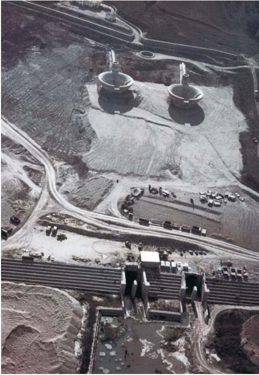
Fig. 48. The morning glory spillways under construction in the eighties at the site of CAMPOLATTARO embankment dam on the Tammaro River, Benevento, Italy
