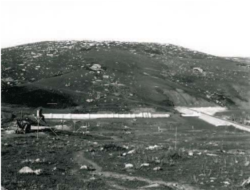
Fig. 116. The TRINITA' embankment dam under construction on the Delia River in Sicily in 1955. The outlet culvert crosses the dam foundation; one can note the reliefs at the extrados in order to improve contact of the concrete with the embankment core material [6] (photo by R. Jappelli, 1955)
